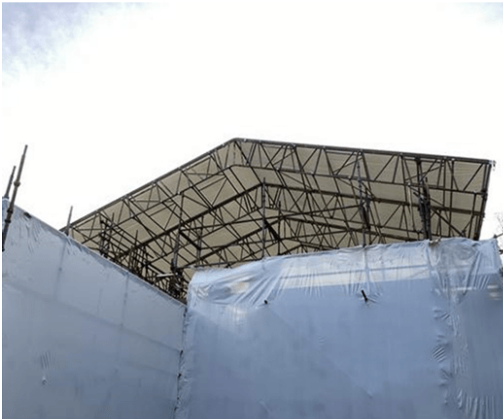
Image 19 CARETAKERS HOUSE: SCAFFOLD AND TEMPORARY ROOF WITH SHRINK- WRAP POLYTHENE SHEETING PROTECTING ONGOING EXTERIOR WORKS.
