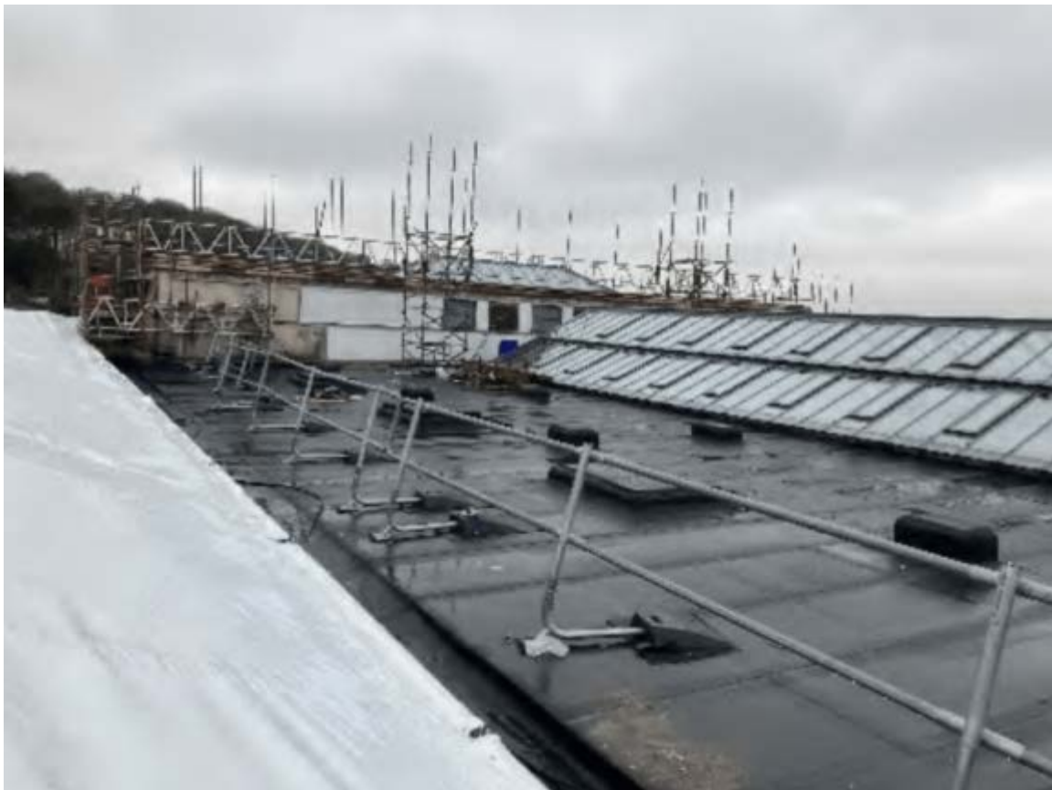
Image 10 ROOF 1 MAIN AUDITORIUM & SKYLIGHT - SCAFFOLDING REMOVED. SCAFFOLD ERECTED AND INSITU FOR TEMPORARY ROOF EDGE PROTECTION.
