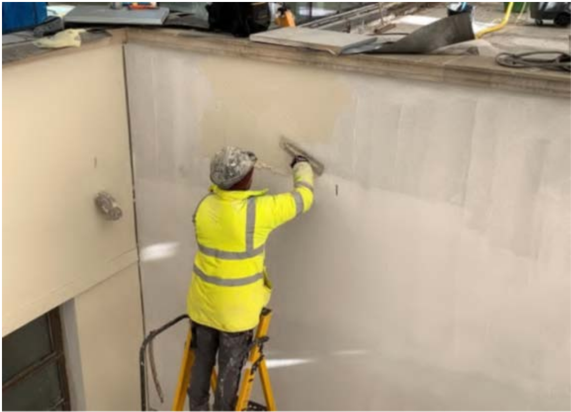
Image 8 ROOF AREA 2E RENDER TOP COAT BEING APPLIED TO EAST AND SOUTH FACING WALL SURROUNDS.
