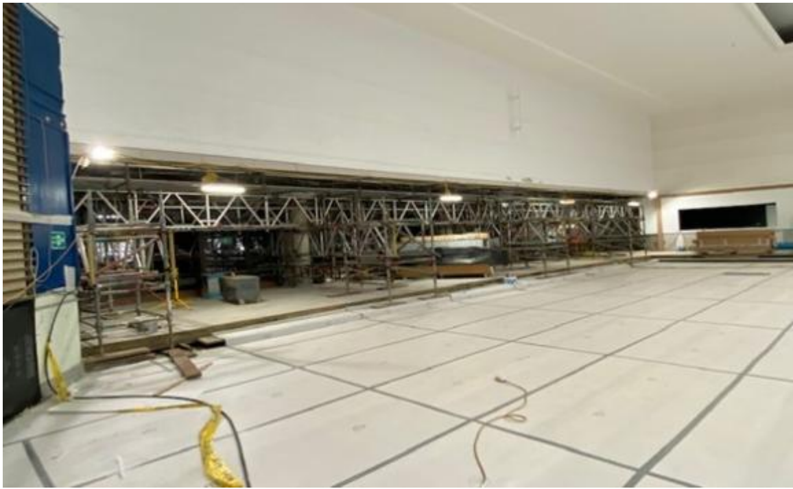
Image 33 MAIN HALL (FRONT ELEVATION/EAST WING): SCAFFOLD REQUIRED INSIDE THE BUILDING TO SUPPORT THE TEMPORARY ROOF FRAME AND BUILDING STRUCTURE.
