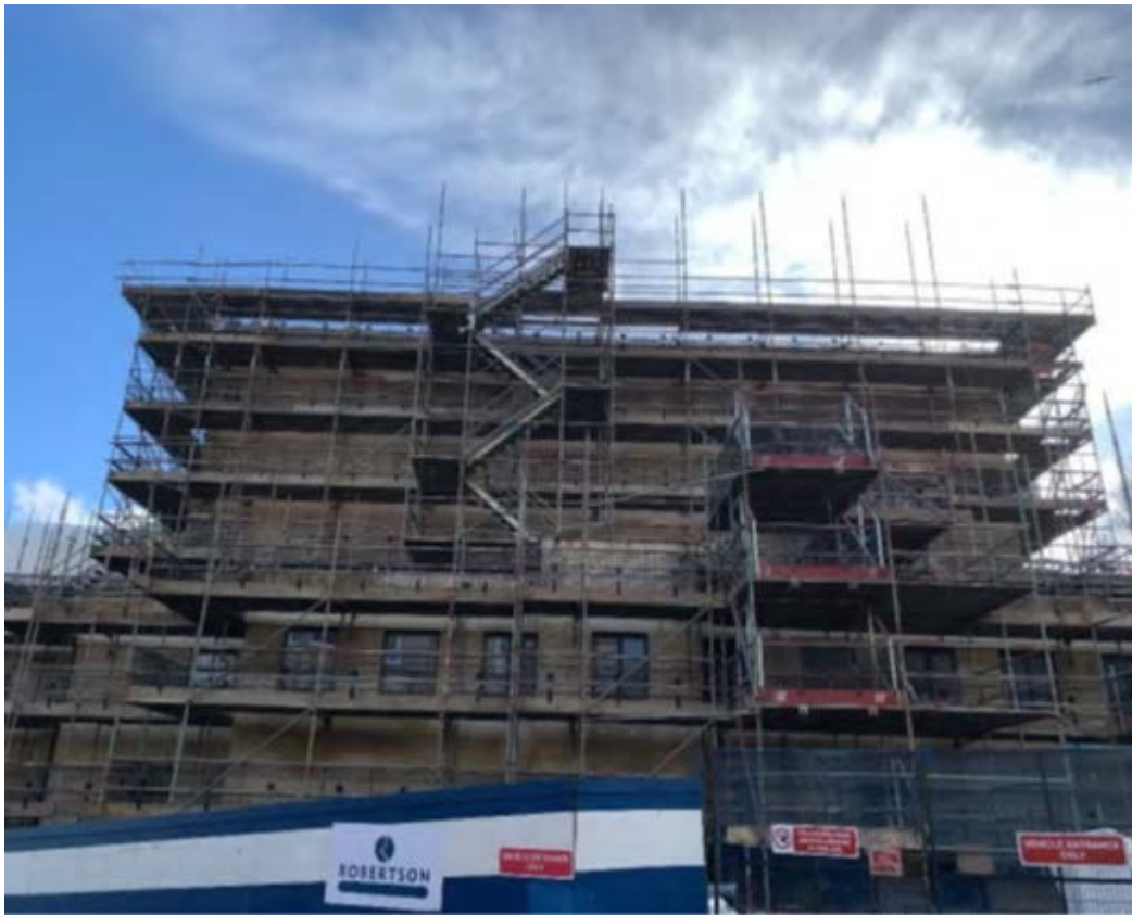
Image 6 NORTH ELEVATION (VIEWED FROM MACKINLAY STREET): SCAFFOLD EXTENDED TO NORTH SIDE OF BUILDING IN PREPARATION FOR TEMPORARY ROOF PROTECTION.
