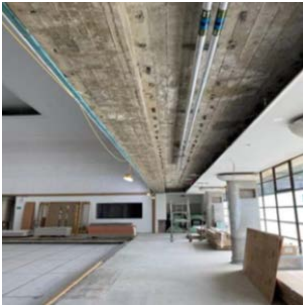
Image 36 PHOTO 3 - MAIN HALL WEST WING: CEILING, MECHANICAL AND ELECTRICAL PLANT REMOVED IN ADVANCE OF SCAFFOLD PROPPING WORKS.
