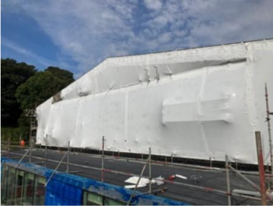
Image 24 MAIN BUILDING: MAIN ROOF (ROOF 1) SCAFFOLD SOUTH FACING ELEVATION WITH SHRINK-WRAP POLYTHENE SHEETING TO TEMPORARY ROOF/SCAFFOLD. OVERLOOKING THE ABUTMENT WITH ROOF 5 FIRST FLOOR OFFICE SUITE.
