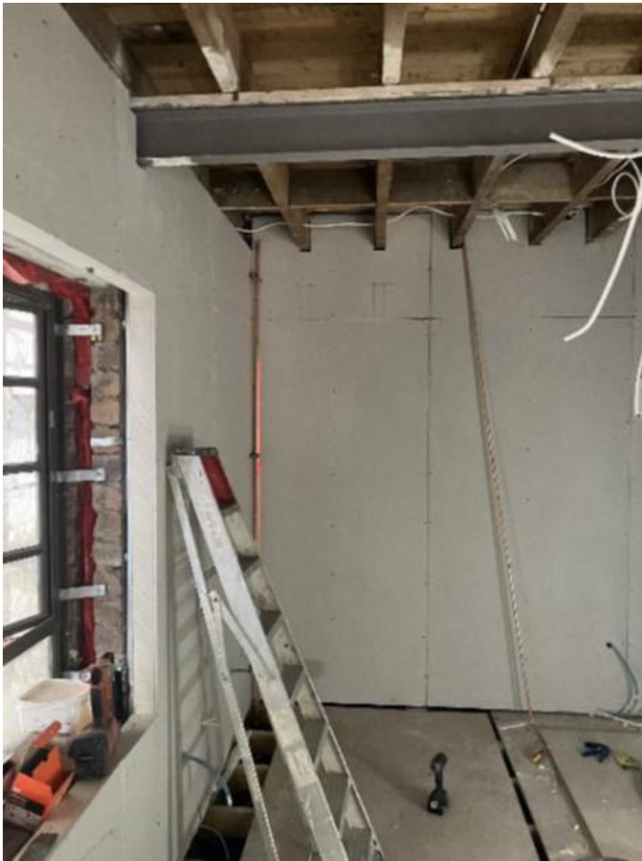
Image 27 CARETAKERS HOUSE: INSTALLATION OF FIRST FIX ELECTRICAL AND INSULATED PLASTERBOARD DRY LINING TO WALLS TO IMPROVE THERMAL RESISTANCE OR ORIGINAL WALLS.
