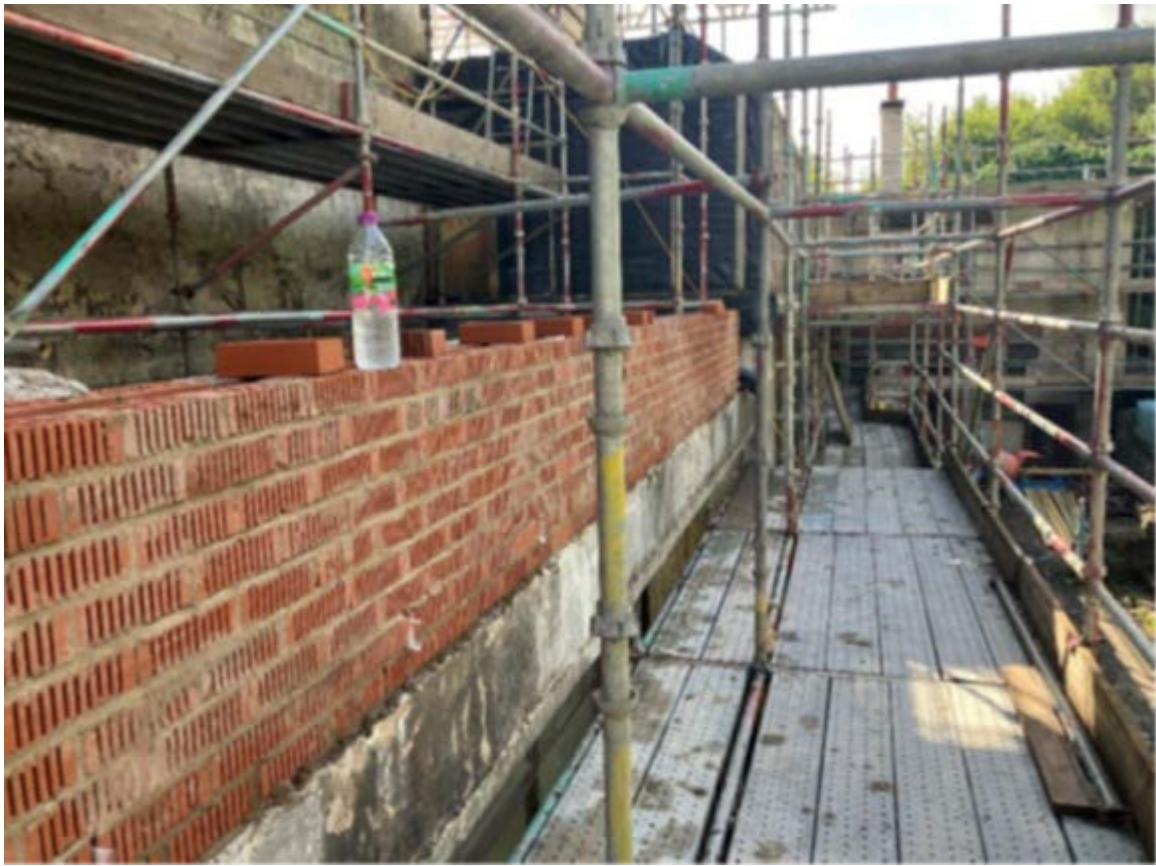
Image 30 WEST ELEVATION: PARAPET UPSTAND TO THE REAR TERRACE ROOF (ROOF 2 SEE PLAN) BEING REBUILT.
