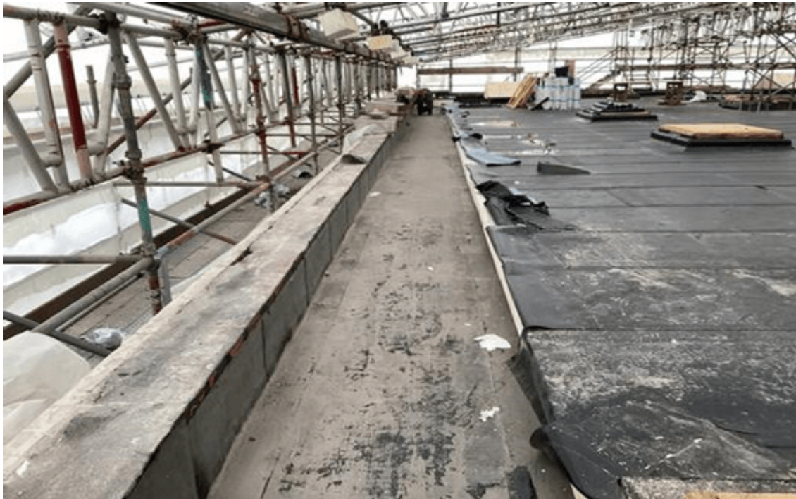
Image 21 MAIN ROOF (1): EAST (FRONT) ELEVATION PARAPET: INSTALLATION OF ROOF MEMBRANE/FLASHINGS TO PARAPET.
