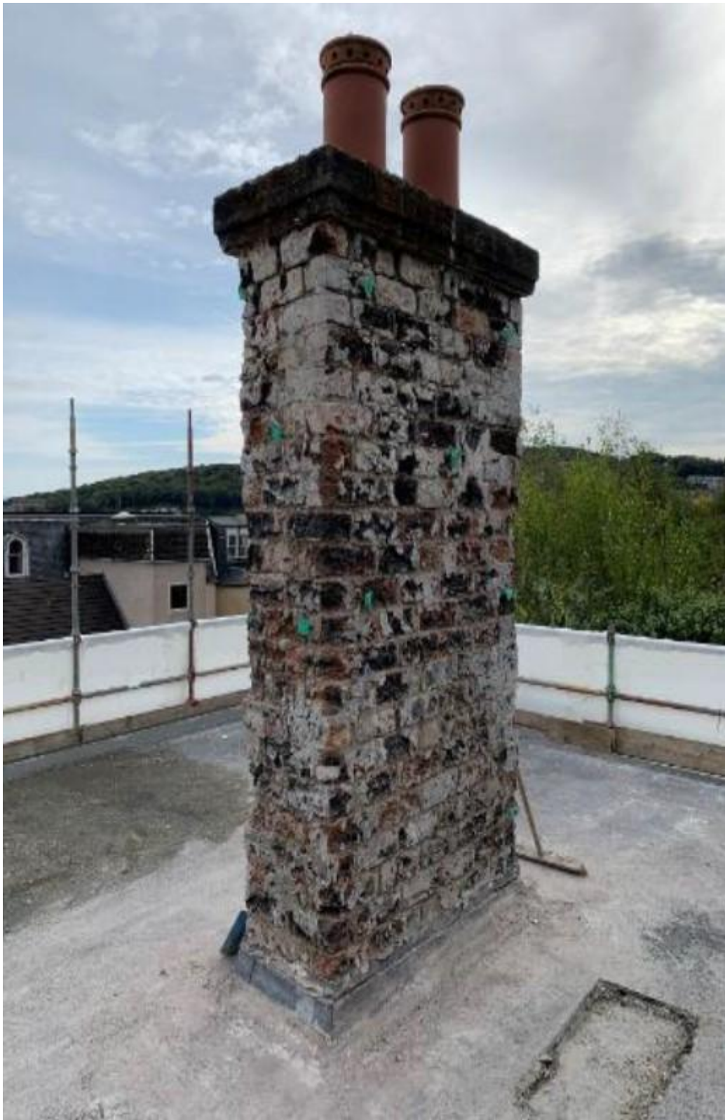
Image 26 RENDER REMOVED FROM THE CARETAKERS HOUSE CHIMNEY.
