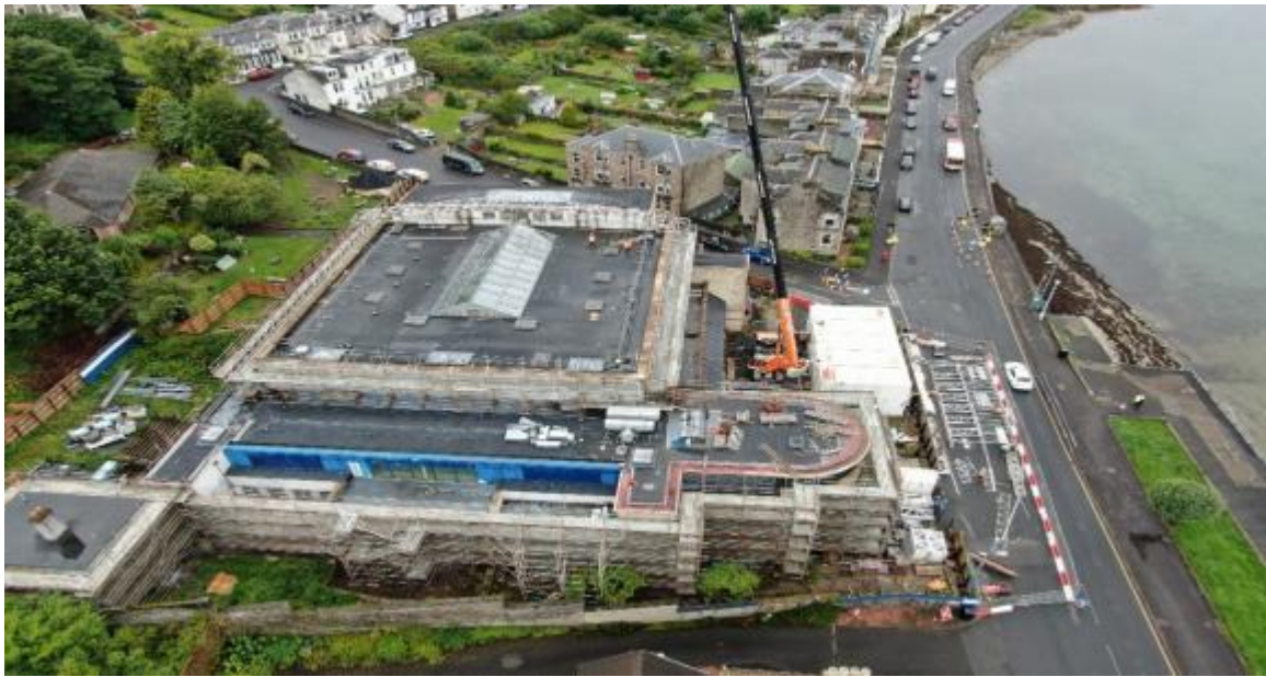
Image 31 ROOFS – MAIN BUILDING AND CARETAKERS HOUSE: FORMED OF 21 FLAT ROOFS ALL AT DIFFERENT LEVELS. ERECTION OF TEMPORARY ROOF FRAME IN PROGRESS – CRANE ON SITE AND PARTIAL ROAD CLOSURE.
