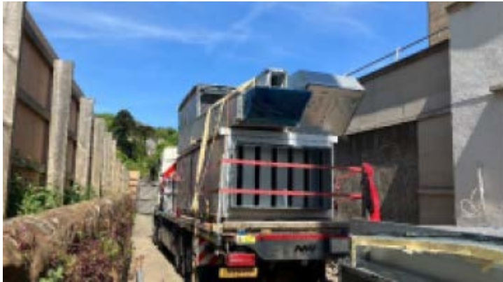
Image 39 MECHANICAL AND ENGINEERING PLANT STORED ON A LORRY FOR REMOVAL FROM SITE.
