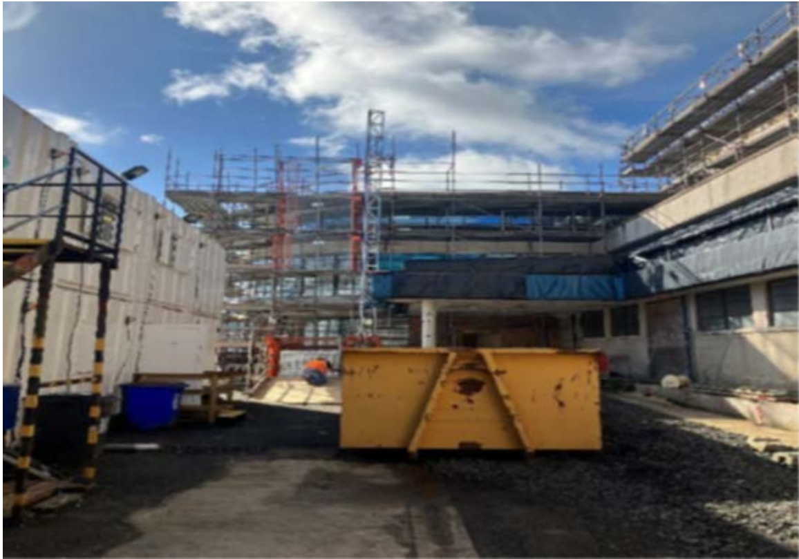
Image 28 MAIN BUILDING: INSTALLATION OF SCAFFOLD LIFT TO EAST ELEVATION OF ROTUNDA IN PREPARATION FOR OVER-ROOF (ROOF 3B).
