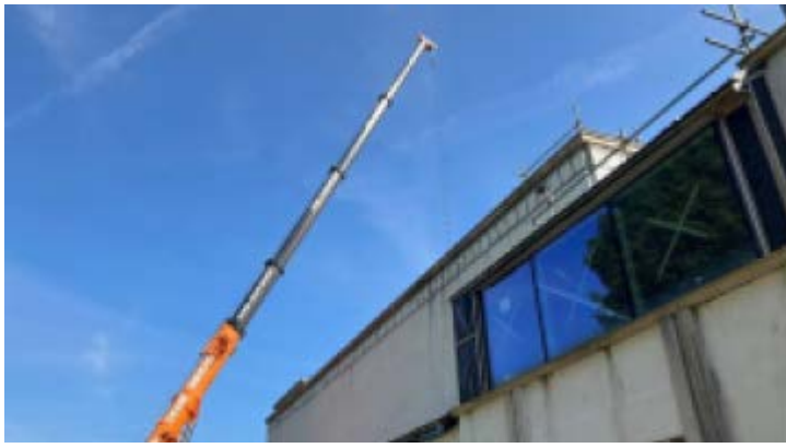
Image 38 MOBILE CRANE ON SITE FOR DISMANTLE OF THE MECHANICAL AND ENGINEERING PLANT FROM THE ROOF.
