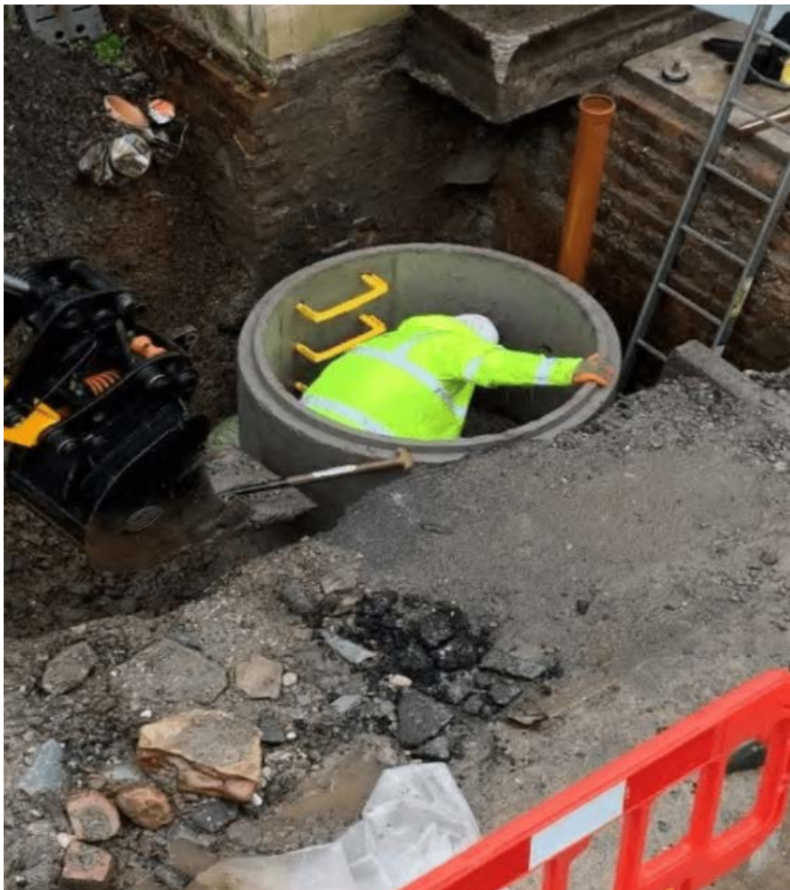
Image 23 (FRONT) ELEVATION: INSTALLATION OF NEW MANHOLE. IN FRONT YARD ADJACENT EXIT FROM STAIRCASE NORTH EAST CORNER OF BUILDING.
