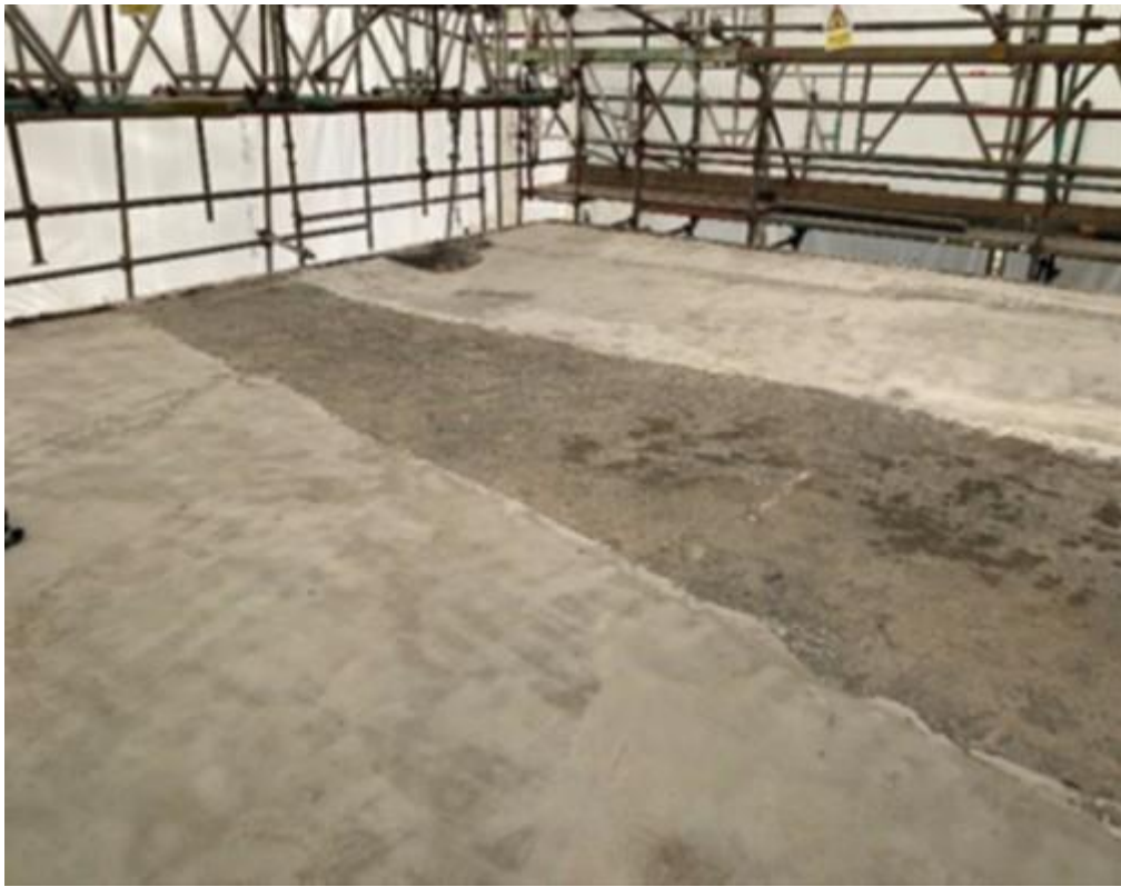
Figure 3 ROOF 3 FLYTOWER: LEVELLING SCREED POURED IN REPAIR AREAS PRIOR TO INSTALLATION OF VAPOUR CONTROL LAYER (VCL).
